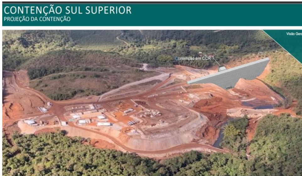
Figure 07 – Construction of the concrete containment located 6 km downstream of the Sul Superior dam, in Baron of Cocais.
