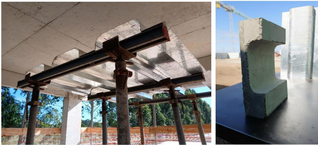
Figure 2 – (A) Arrangement of metal forms in the shoring; (B) Full-scale prototype of the H12 mini-slab after formwork removal.
