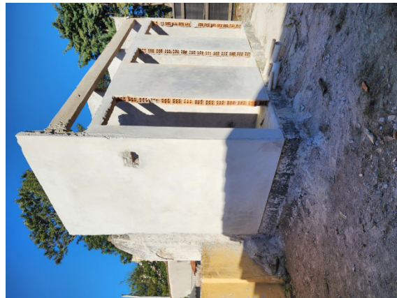
Situation registered in May 2023. Bathroom structure already built with beams and plumbing. apparent ment
